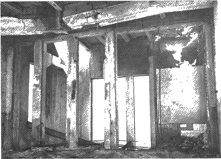
Figure 5.20a. Upper photo: Reinforced-concrete, aseismic structure; window fire shutters were blown in by blast and the interior gutted by fire (0.12 mile from ground zero at Hiroshima). Lower photo: Burned out interior of similar structure.
